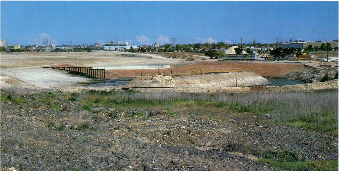
Construction of the artificial lake and island in the southern section of the park (see plan). Photo: J. Fields
